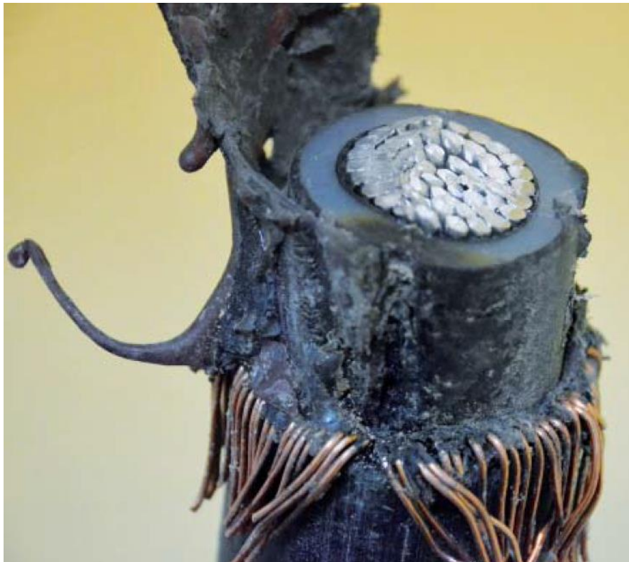
Figure. Single-core 10 kV cable after removing parts of the damaged coupling from it.
