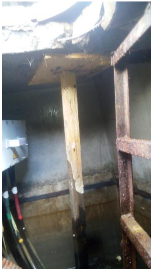
Photo 3. The collapse of the ceiling of a concrete well.
