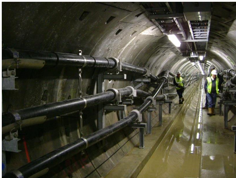
Photo 1. Transposition of the single-core cables themselves.
