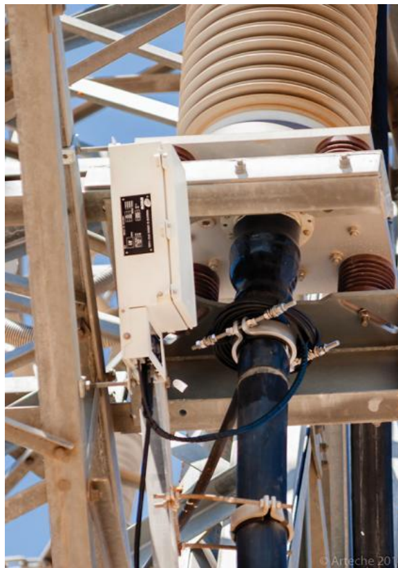
Fig.13. Measuring loop of the optical CT mounted on the cable under the termination
