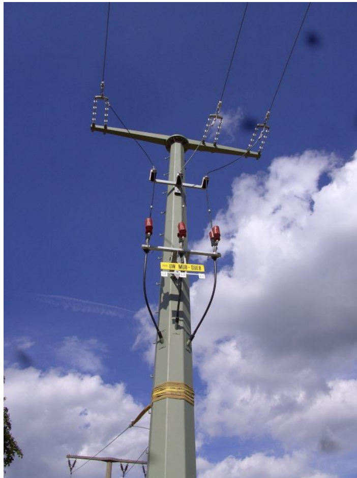
Fig.9. TP on an OHL tower (steel pole). The cable runs inside the tower
