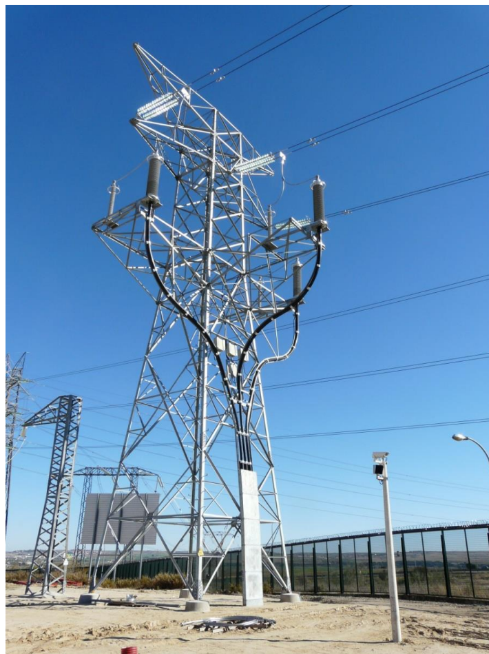
Fig.3. Double-circuit TP on the OHL tower (lattice)
