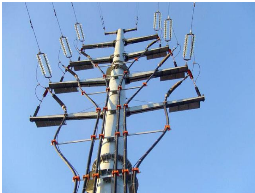
Fig.7. TP on a double-circuit OHL tower (steel pole). Dry flexible terminations are used
