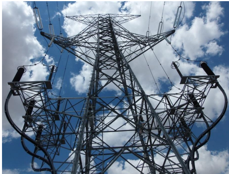
Fig.4. Single-circuit TP on the OHL tower (lattice)
