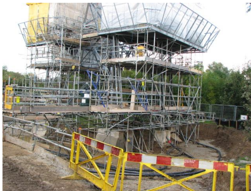
Fig.5. Construction of scaffolding around the TP, made on the OHL tower, for the subsequent installation of cable terminations
