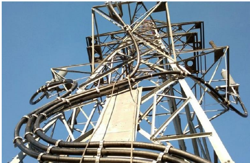
Fig.10. TP on an OHL tower (lattice). The cable stock is equipped on the tower body
