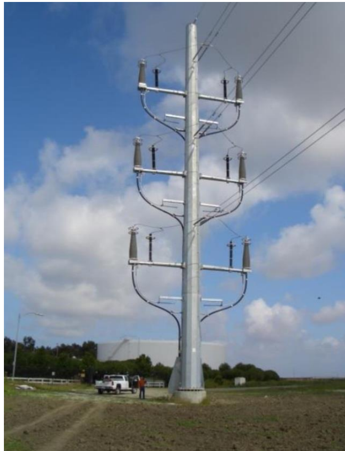
Fig.8. TP on an OHL tower (steel pole) having two cables for each phase of the OHL
