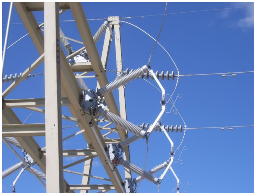
Fig.11. 115 kV class TP equipped with a V-shaped disconnector
