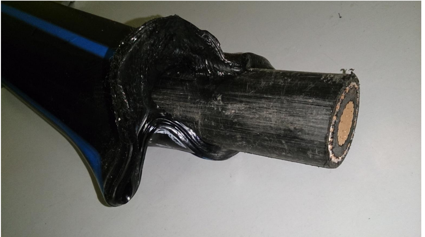
Fig.6. Deformation of the HDPE pipe and pinching of the single-core cable laid in it.
