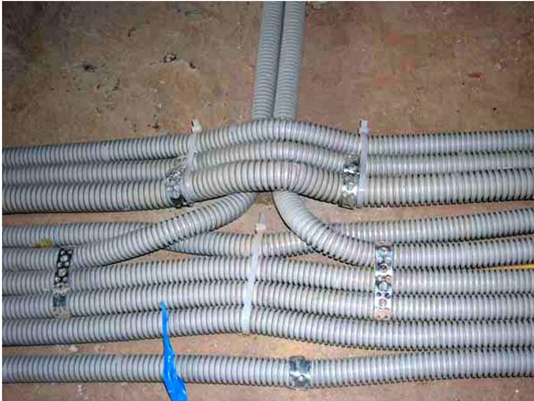
Fig.2. Electrical wiring 0.4 kV made of corrugated pipes.
