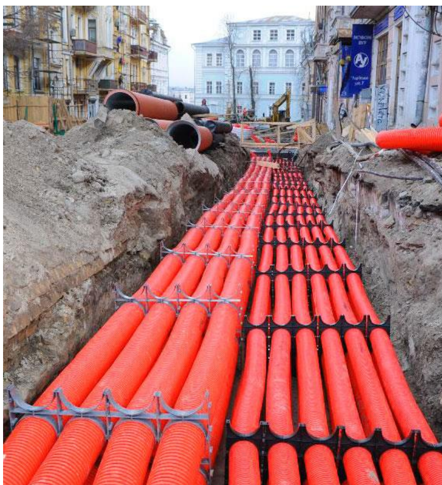
Fig.5. 0.4 kV cable lines laid in a double-walled corrugated pipe and located in a trench.
