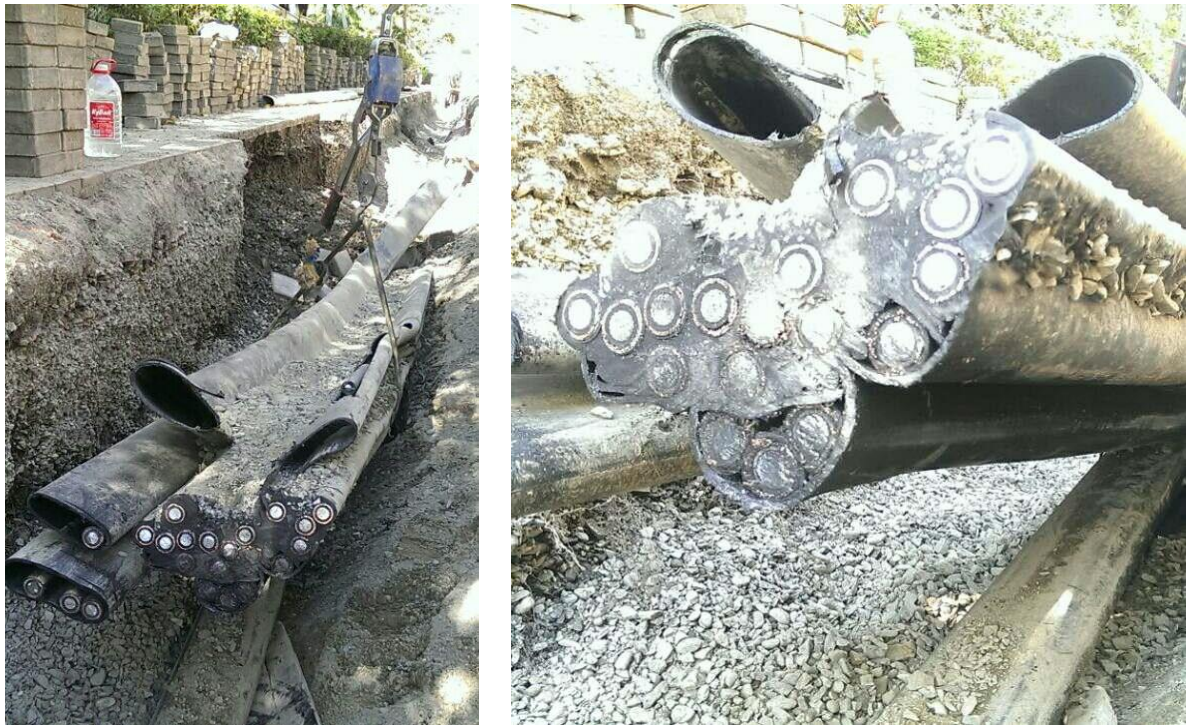
Fig.1. Consequences of negligent attitude to laying cables in pipes.
