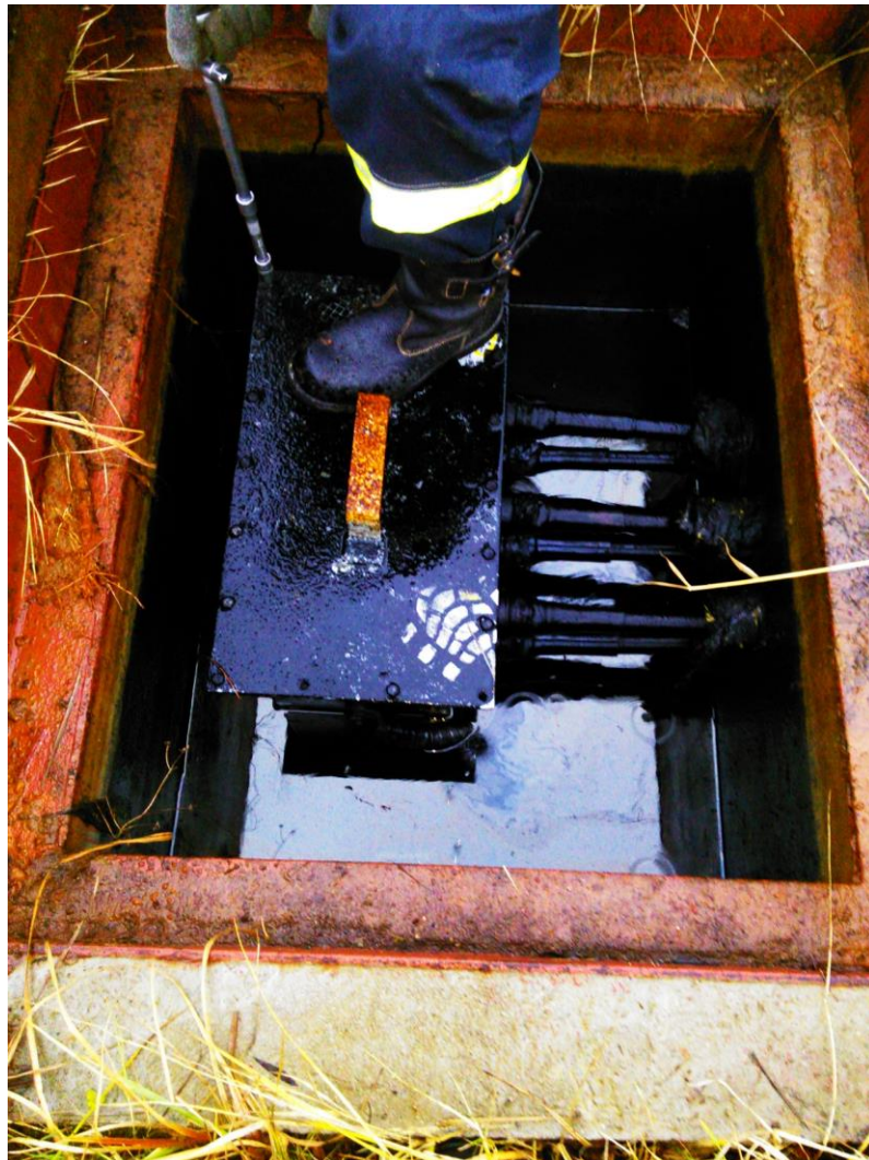
Fig.6. The process of opening the link box in the "compact" concrete well.
