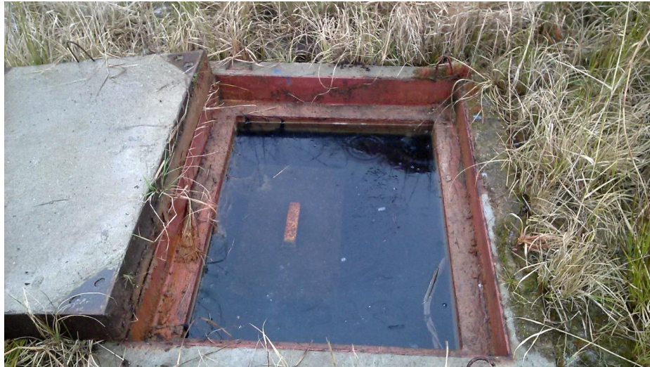
Fig.5. A link box installed in a "compact" concrete well.
