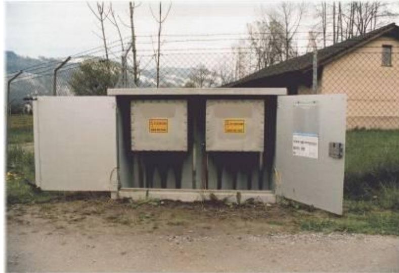
Fig.1. Placement of screen cross-bonding boxes in outdoor structures.
