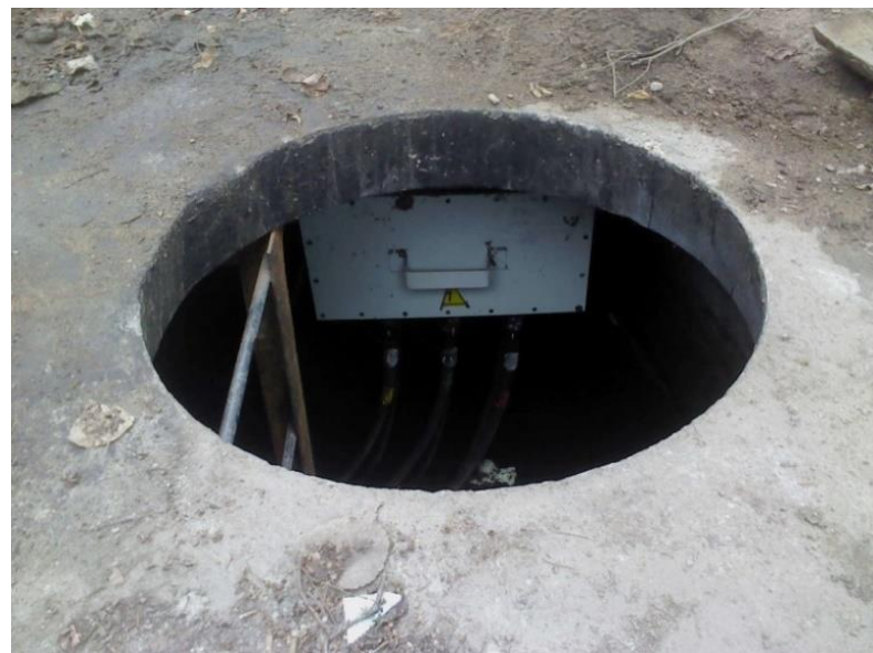
Fig.2. Placement of boxes in the upper part of the underground concrete well.
