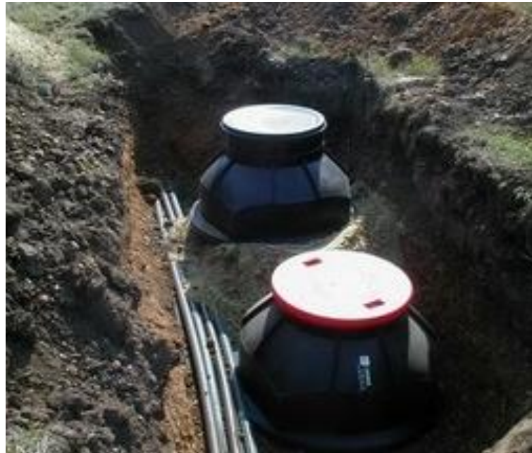
Fig.3. A cross-bonding well with the use of concrete ring and a plastic neck.
