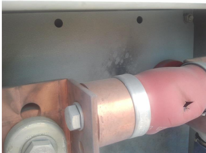
Photo 2. The consequences of using a 3 kV MOA in screens end link-box (ELB) of foreign production.
