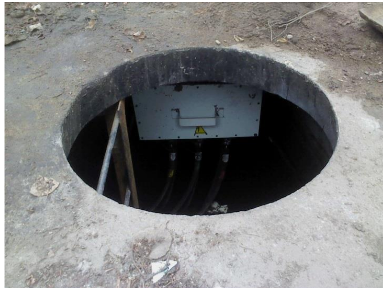
Photo 3. A cross-bonding link-box with two bolts instead of 18, placed in the upper part of the well.
