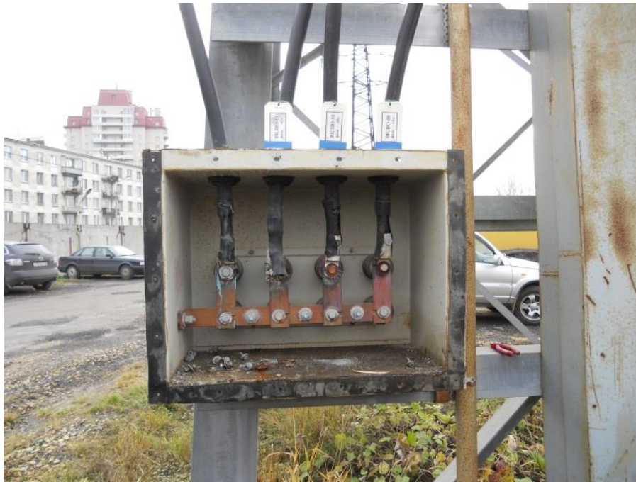
Photo 1. The end link-box, where connecting wires pass from upper surface and the Cu-Al pair applied. Due to the ingress of water and electrochemical processes, screens of phases "A" and "B" burned off from the grounding bus.
