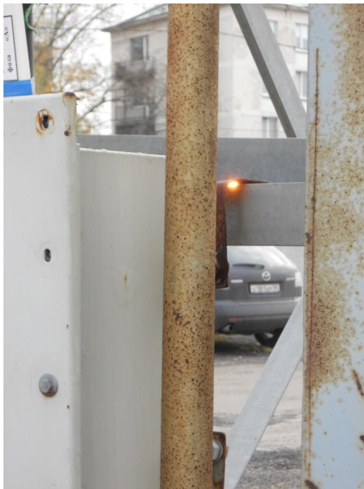
Photo 2. Damaged end link-box (Photo 1) in the parking lot. From the housing through the arc to the body of the tower and then into the ground flows the current of the screen phase "C", which is about 50-100 A.
