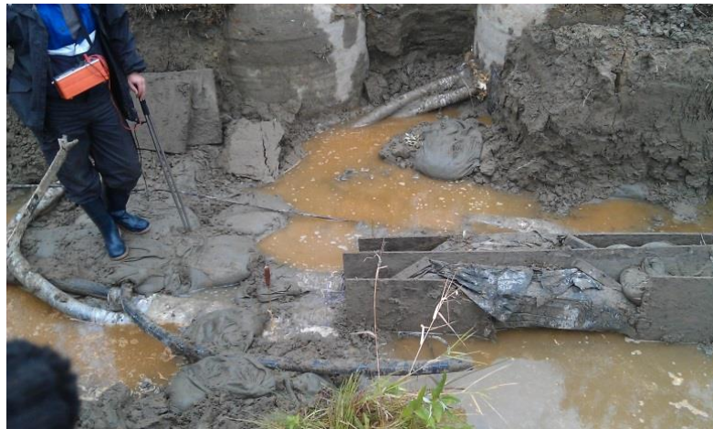
Photo 5. Homemade cross-bonding of 110 kV cable joint – plywood boxes filled with silicone and wrapped with polymer wrap.
