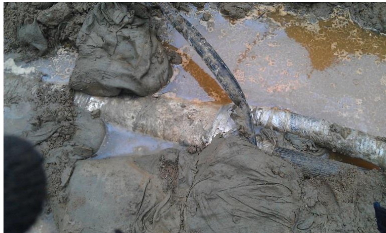
Photo 4. Homemade cross-bonding 110 kV joint. The phase of the cable is shown; the coaxial connecting wire outputs screens to outside; the scotch tape with which the place of screens output and the coaxial wire are wound. The third cable with a crease is visible from above – the output of screens of another phase.
