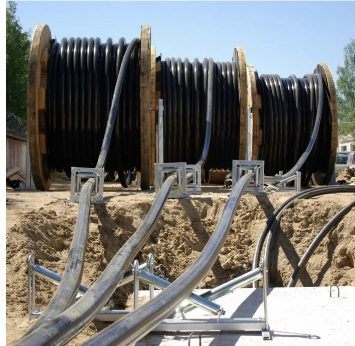
Underground cable line (CL)
