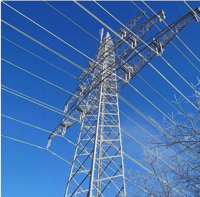
Overhead line (OHL)
